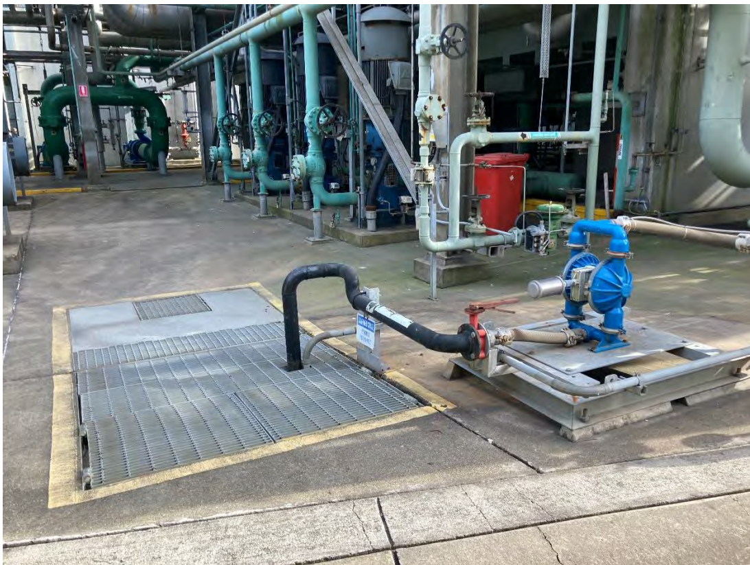
Figure 12 Steam turbine area collection pit and pump
