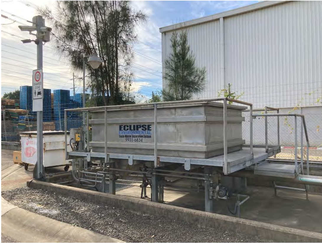
Figure 5 Eastern SEF boundary 30kL/hr oil water separator
