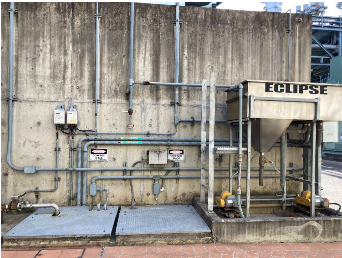
Figure 2 Southern SEF boundary 3kL/hr oil water separator
