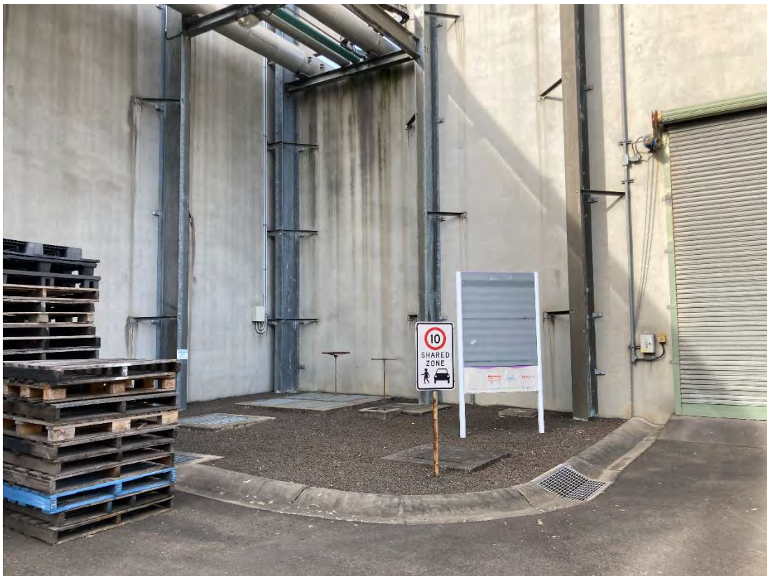
Figure 4 Southern SEF outlet control pit and vehicle roller shutter door
