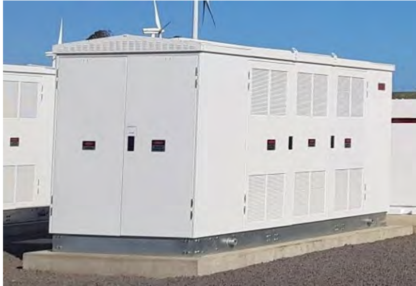
Figure 4-4: Example of transformer
