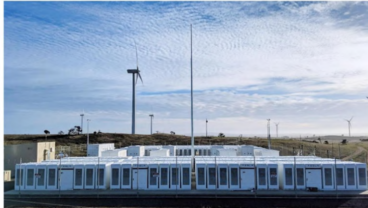
Figure 2 - Lake Bonney Battery in South Australia
