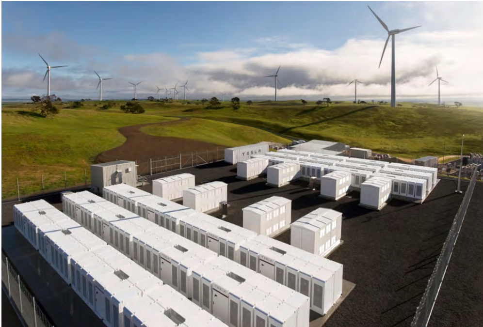
Figure 3-1: Example of a BESS (Lake Bonney Wind Farm)
