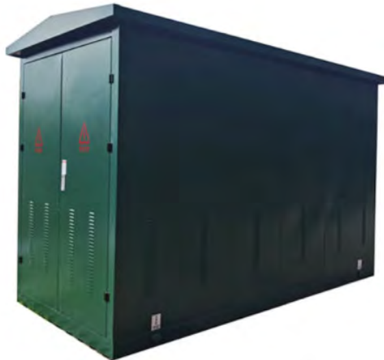
Figure 4-5: Example outdoor switch room
